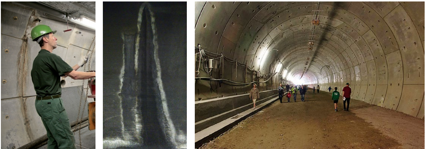
Figure 4-9: Salt deposits at joints of concrete segments in the Belgian URF (left) and Dutch traffic tunnels - Westerschelde (middle) with whitish deposits and Sluiskil (right) with joints between segments in the top, no salt deposits yet. All tunnels have been constructed in Boom (Rupel) Clay.
