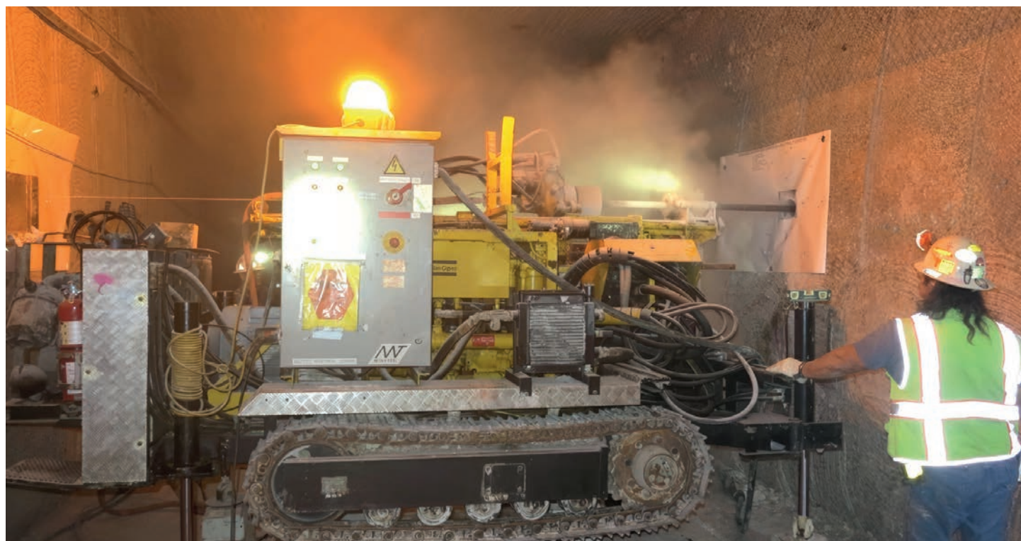
Figure 2.8) A borehole is drilled into the wall of the WIPP for experimental purposes. Source: Kristopher Kuhlman, Sandia
