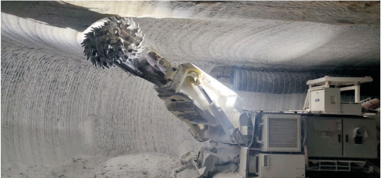
Figure 2.4) A road header used in a salt mine. Photo by Jeroen Bartol, COVRA
